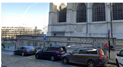
Balustrade existante – photo Streetview
